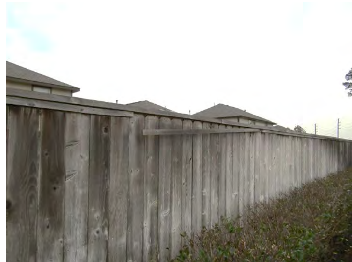
loose trim piece
